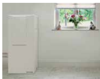
Oil boiler fitted internally with Grant plume diverter utilised for flue (Part code: VTXBFAIR/VTXBFAIR2)
